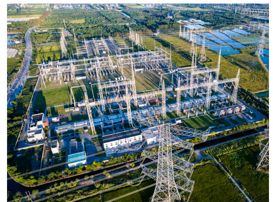
Aerial view of electricity pylons and a big electrical substation at Shanghai city, China (Getty Images)
